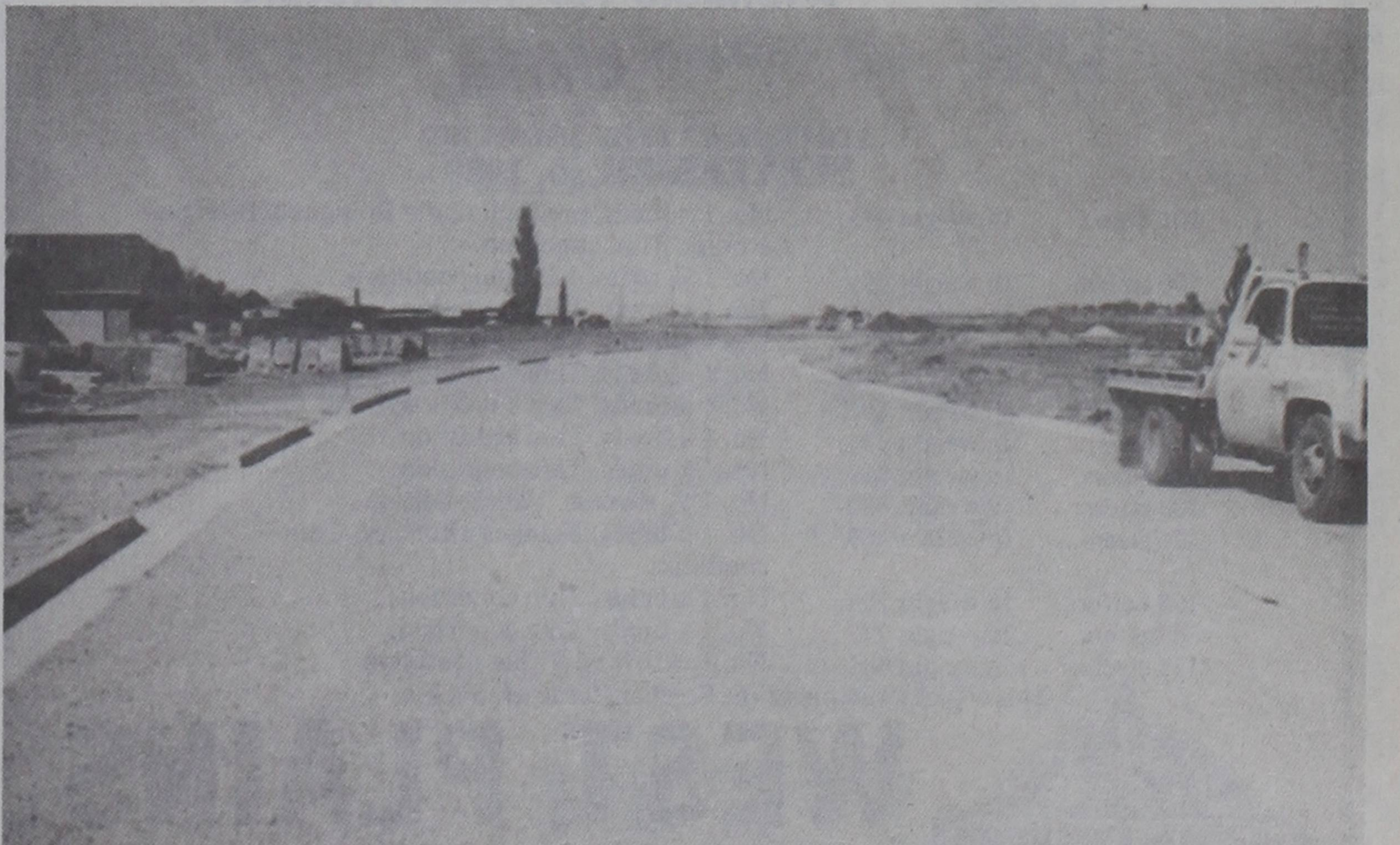
STREET PAVED... North Springfield Avenue was paved this week. This is the street on which the new homes are under construction by Reata Land Company. The first four homes in the project are well underway, and are nearing completion. Good weather in recent days has aided the progress on the new project.
