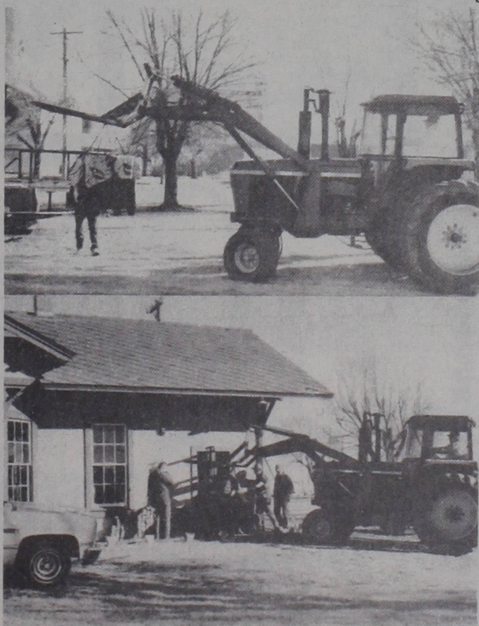
LOADING.... Mark Osborn mans the front-end loader as the safe was moved into the Depot last week.
