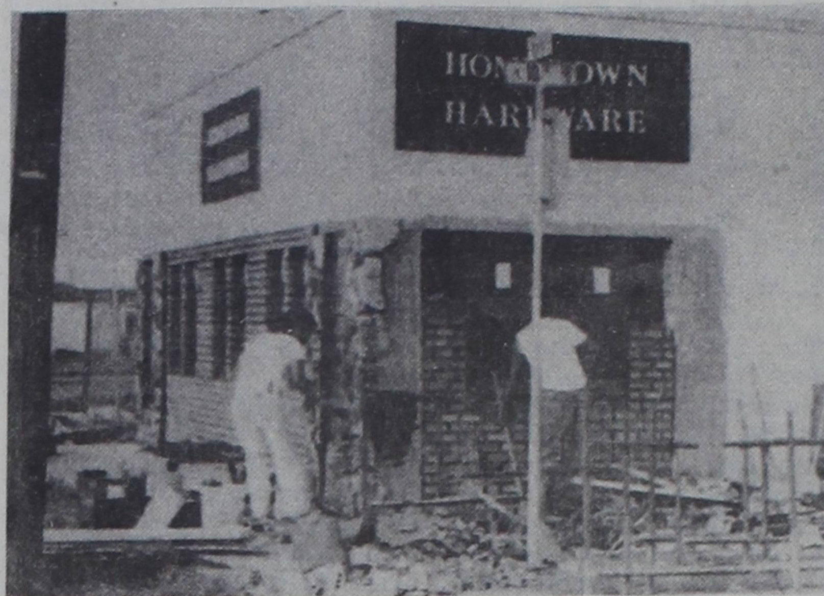
REPAIR WORK...Workmen are shown putting in a new front at Hometown Hardware, whose building was damaged recently by an out-of-control vehicle.
