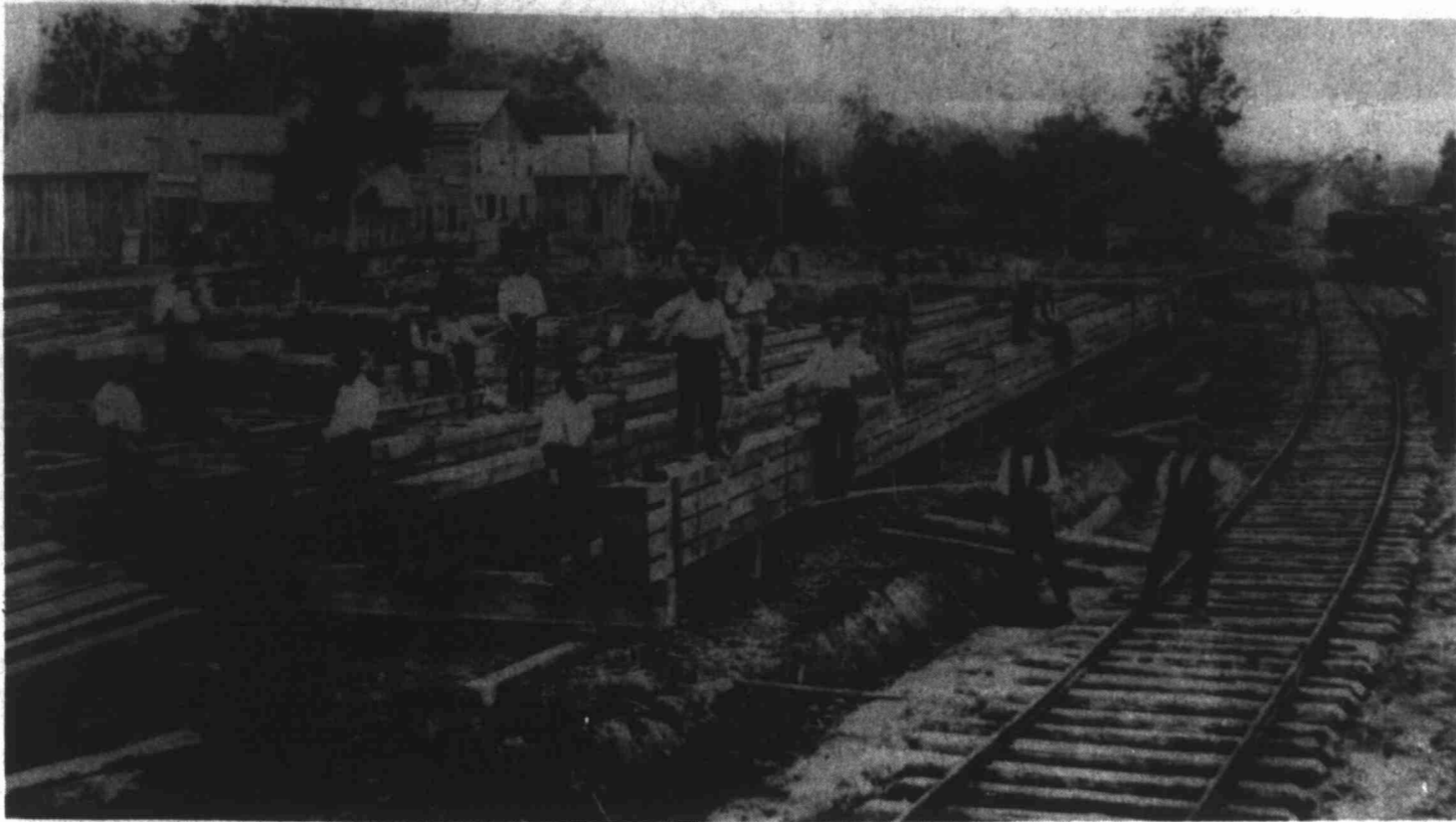
MUSCLE WAS DRIVING FORCE — Early-day railroad construction lacked the refinements which have become an essential part of the industry today. Brawn was the driving force for getting the work done as
