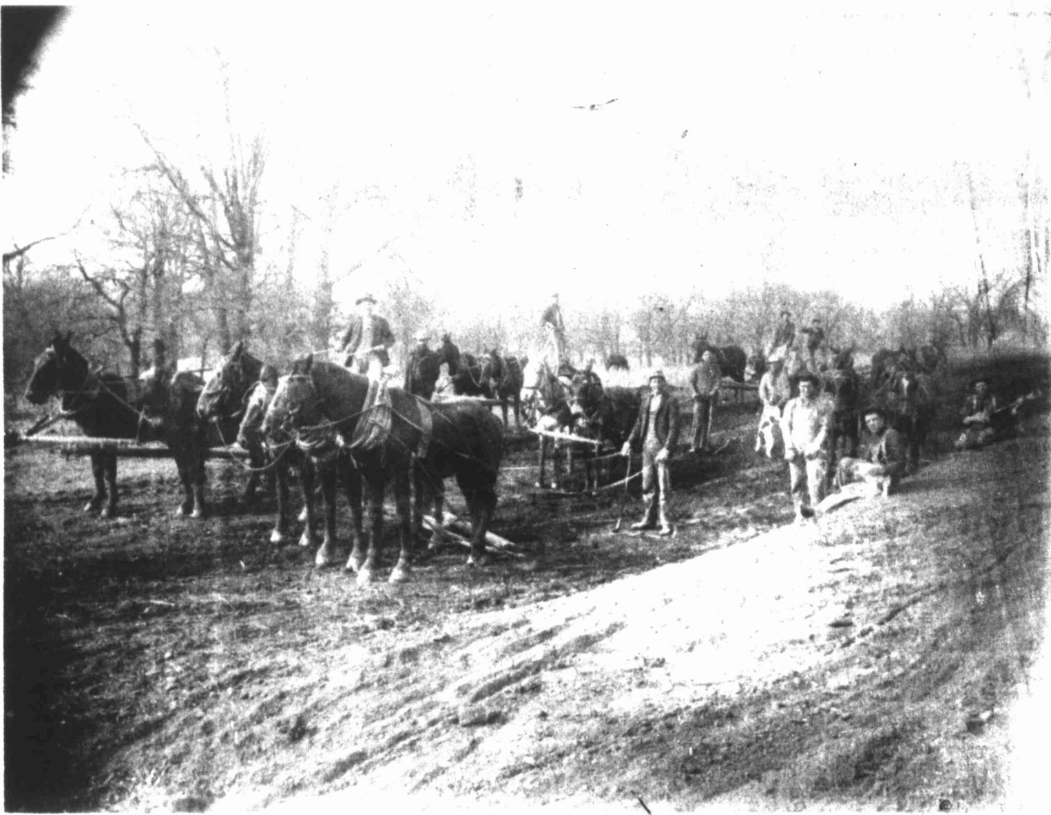
CLEARING A THOROUGHFARE — These crews were clearing the right-of-way for the old Bankhead Highway through the middle of the old Cottonwood Park in the early part of the century. The horses and mules did their part to hasten the arrival of the 'horseless carriages' into Big Spring. The roadway being clear is now East Third street near Birdwell Lane.
