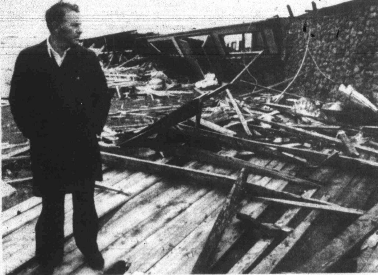
CHURCH DESTROYED — The Rev. Bill McClellan of the Liberty Heights Free Will Baptist Church, looks at the remains of the structure Monday after a tornado ripped through the south Tulsa suburb Sunday while an Easter service was in progress.
