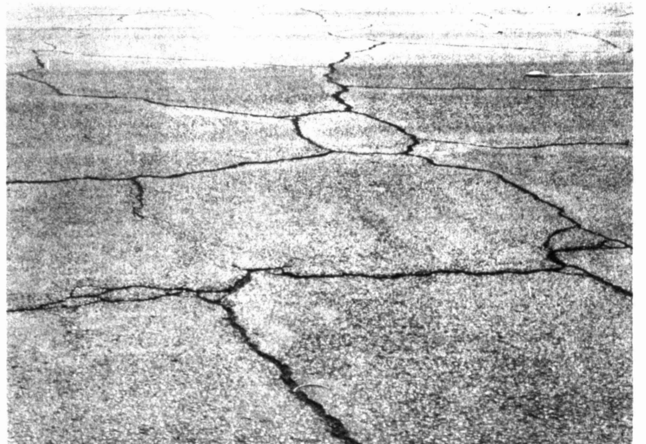
TELLTALE SIGNS OF A PROBLEM — Many streets in Big Spring are showing grave signs of wear and tear. The cracks in the pavement here are indications that the thoroughfares are crumbling away. It's estimated some 600 blocks of streets within the system are beyond repair. The voters get a chance to do something about the problem in a bond election scheduled here Dec. 13. Total amount proposed for all street improvements is $4,545,000. Voters will determine the fate of each of nine capital projects improvements by casting ballots on each individually.
