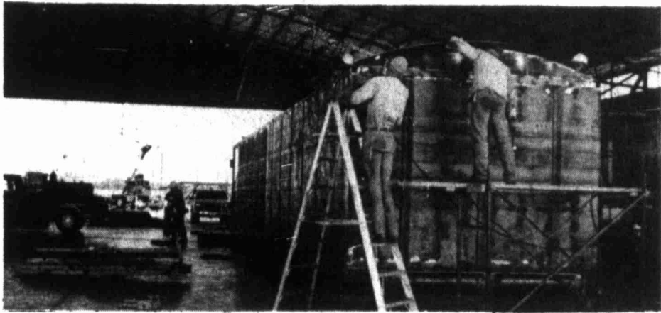
WORKERS AT LOCAL FIRM ASSEMBLING 'DOG HOUSE' This building will fit onto sub-structure of oil derrick
