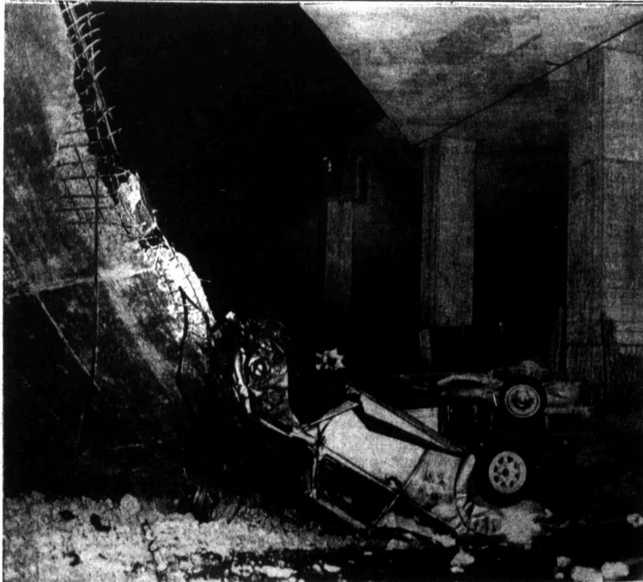
NORTHCOAST EARTHQUAKE — A passenger car and a light truck fell more than 30 feet when a Highway 101 overpass 8 miles south of Eureka, Calif., gave way during an earthquake early Saturday morning. Six people were
