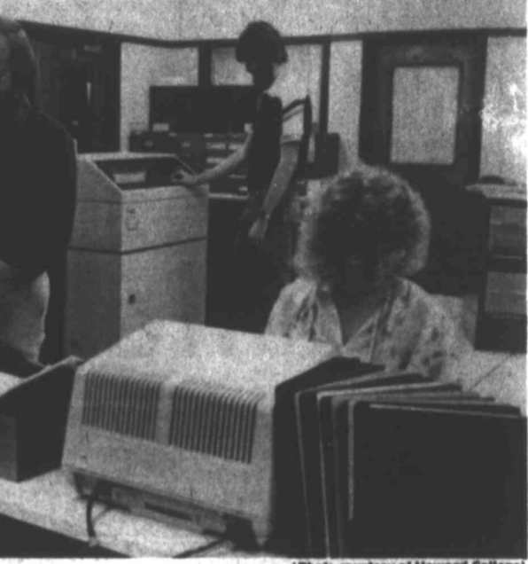
PROGRESS — Terry Hansen, left, Tony Claxton, background, and Joy Vaughn, work on the new computer at Howard College. The computer was recently installed and has greatly increased the capacity of the data center. Claxton is one of two new teachers in the computer program at HC. Hansen is now an instructor as well as the director of the computer center.
