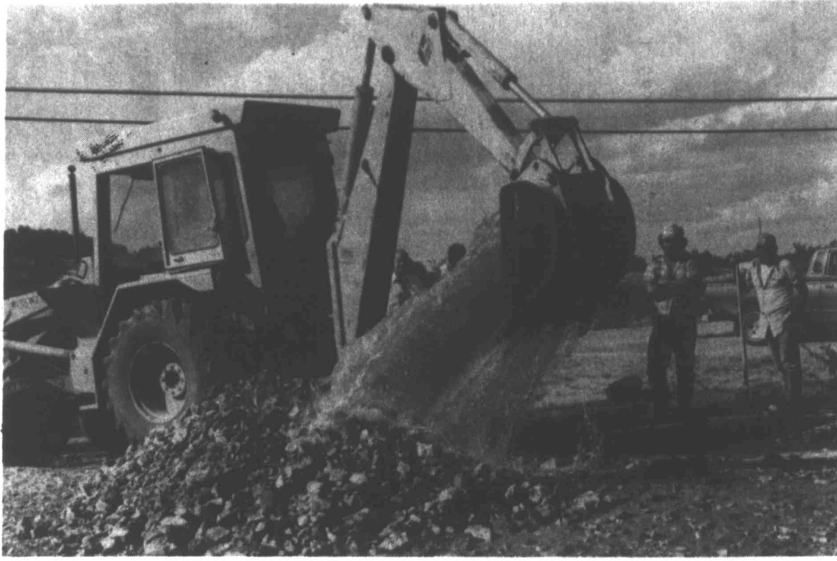
ARID AREA — Residents in the Wasson addition and others living in the southwestern portions of the city had to get along without water for several hours Tuesday as city workers worked to stop a major leak in a pipe along Thorp Road. The situation here has deteriorated to the
