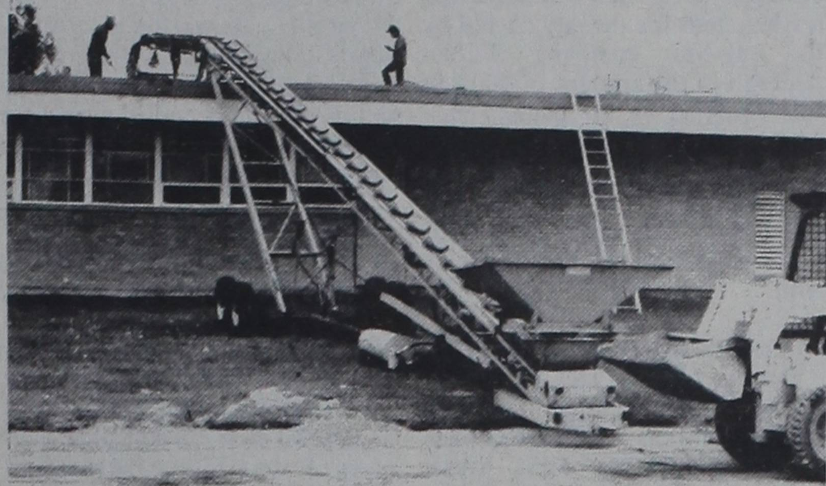
HIGH SCHOOL WORK... Workmen are shown re-roofing the high school building following the damaging hailstorm of last month. The high school's roof was badly damaged by the hail.
