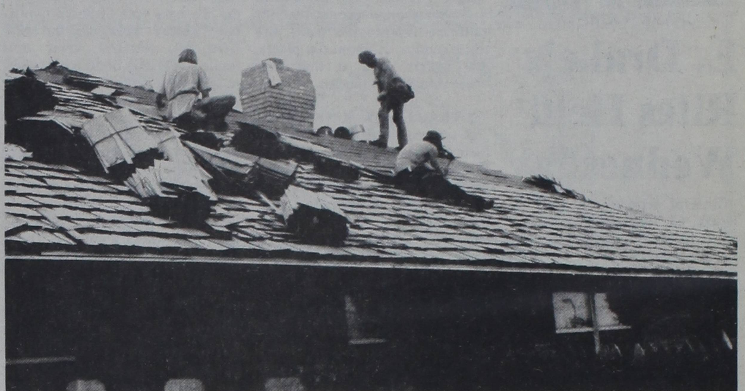
ROOF WORK... Workmen on top of houses has been a common sight in Friona during the past couple weeks, due to damage from the big May hailstorm. In the above picture, workers are shown re-roofing the home of Mr. and Mrs. D.L. Harguess, 1604 West Tenth Street.
