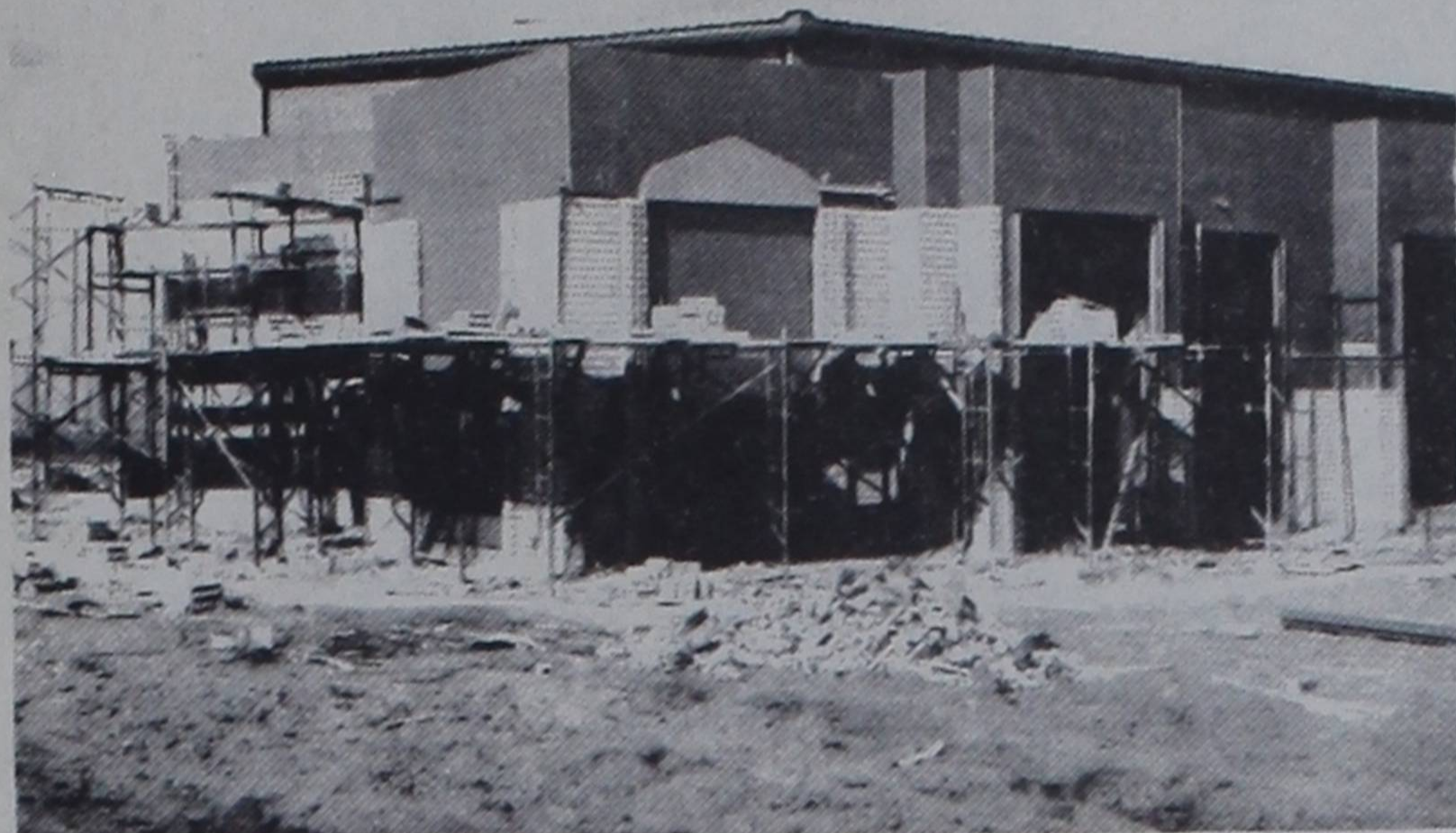
TAKING SHAPE... The new sanctuary for Calvary Baptist Church is beginning to take shape in the northern part of town.
