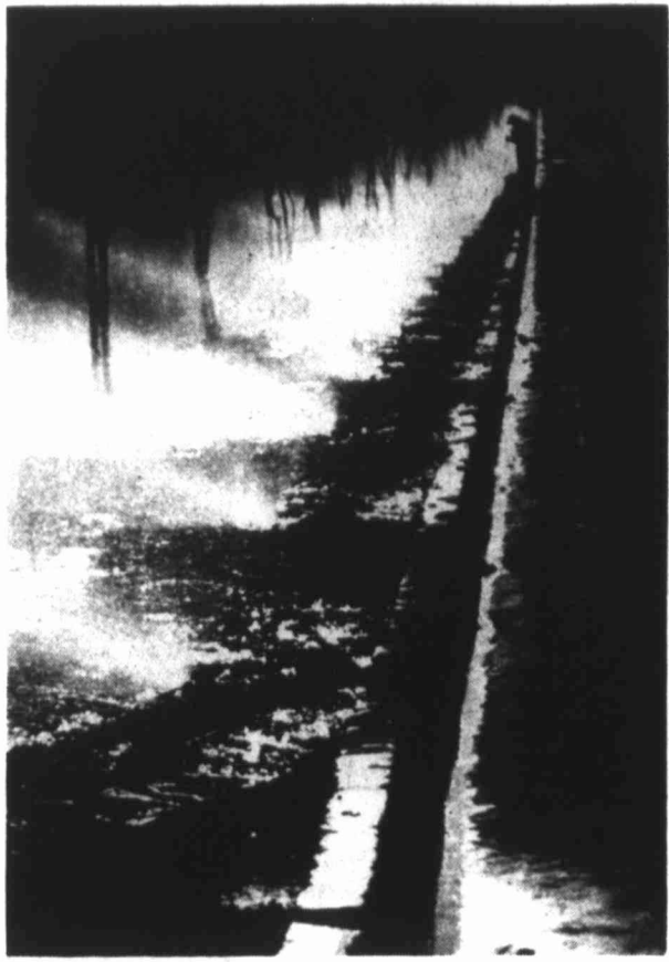
EARLY MORNING SPRINKLE — Sunlight filters through the spray of a newly installed sprinkler system on Gilmer Road in Longview recently. This early morning shot caught a construction worker cleaning the street shortly after helping install the sprinkler at an entrance to a neighborhood development.
