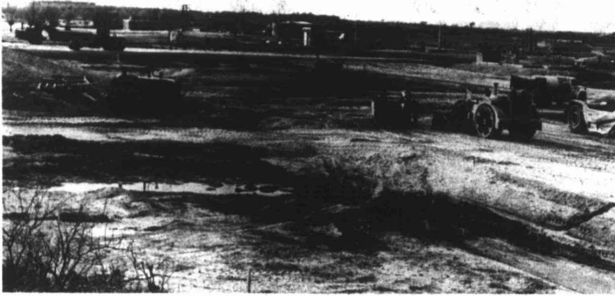
FUTURE FOUNTAINS — Work has begun at the Big Spring Sewage Treatment Plant on the construction of two aeration ponds. According to City Manager Don Davis, the ponds will be "fountain-like," and will spray water into the air in order to oxidize contaminants. The crews pictured are grading the area to be used for the ponds.
