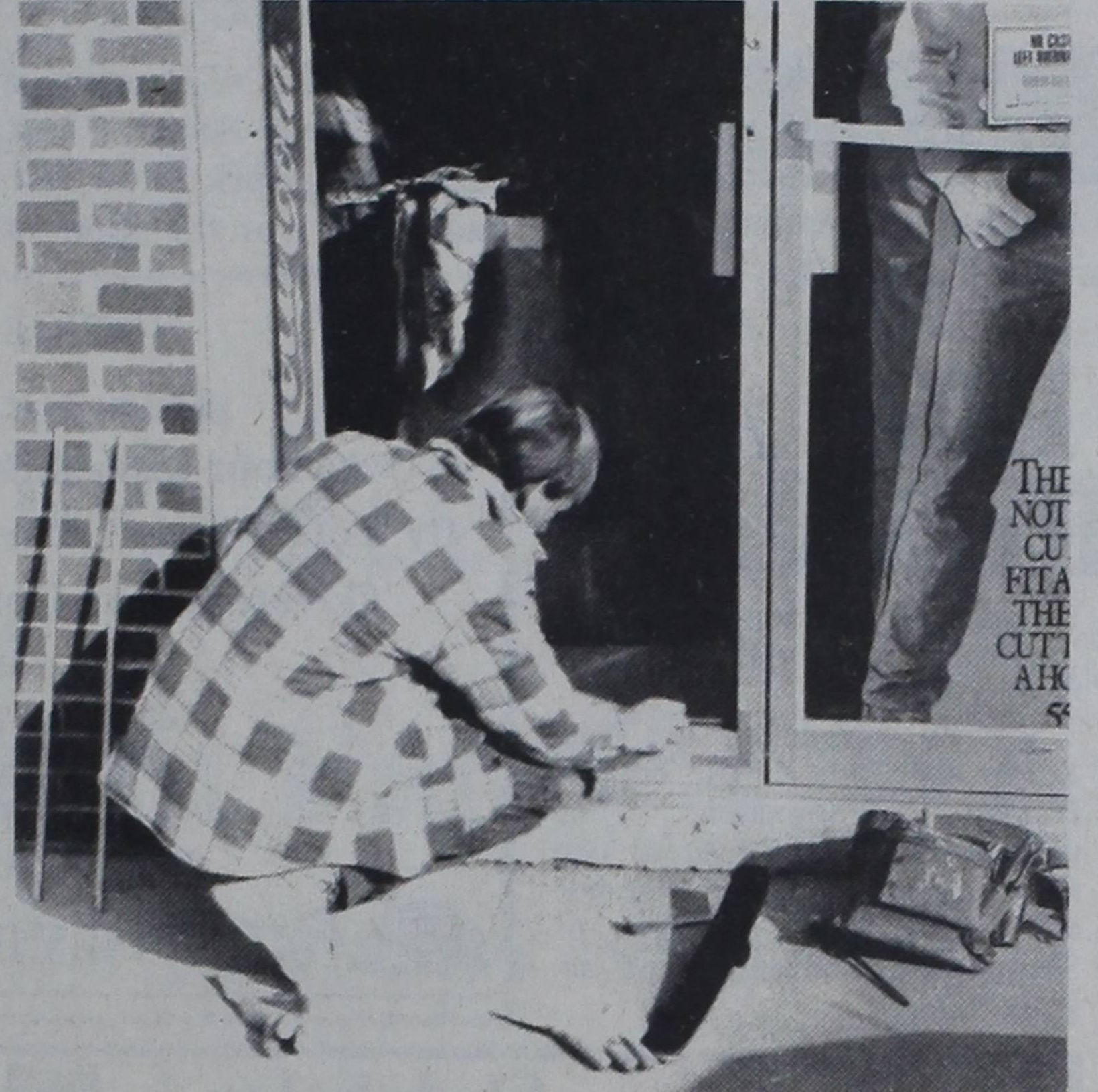
BREAK-IN REPAIRED... A glass company employee is shown making repairs at Malouf's in Friona following the break-in sometime Wednesday night. Burglars took an undetermined amount of ready-to-wear, including jeans, coats, hats and boots.
