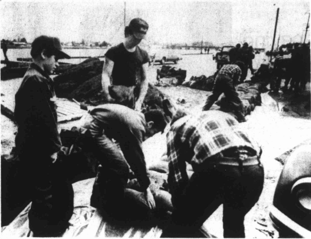
GETTING READY — Emergency crews and members of the civil air patrol build a wall of sandbags Tuesday between the Skagit River and Mount Vernon, Wash., as
