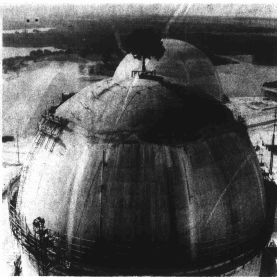
TREE TOPPING — A cedar tree, about 27 feet tall, was lifted atop the 160-foot-high dome of the Comanche Peak nuclear plant's Unit 2 reactor containment building to mark the completion of concrete placement on the exterior of the building. Unit 1, which was topped out last January, is in the background.
