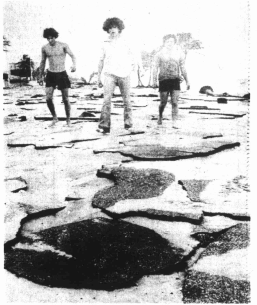
ROUGH ROAD — Ft. Lauderdale residents Marc Berson, Randy Cooper and Jeff Forem (left to right) walk gently over portions of State Road AJA in Ft. Lauderdale Monday. The Damage to the road was caused by high winds and surf from Hurricane David.
