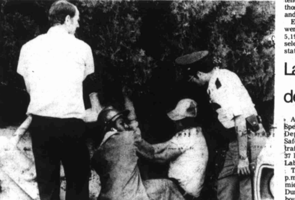
BROKEN GAS LINE — A broken gas line was fixed Monday morning at 6th and Birdwell after it was struck by a garbage truck. The truck had no damage. Fixing the pipe are (from left) Ike Wasson, Willie Rabb, Stan Thornton and Joe Diliberto.
