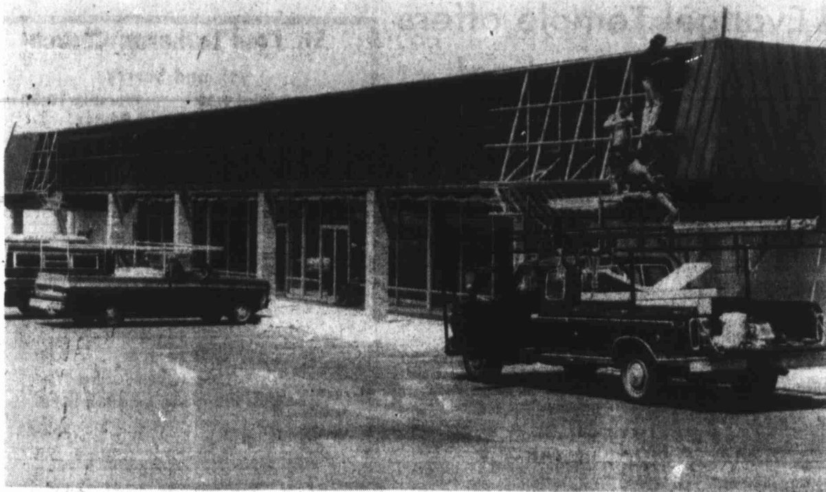
MOVING AHEAD — Construction is moving steadily ahead on the new location of the TG&Y store in the College Park Shopping Center in East Big Spring. The spacious structure should be ready for occupancy sometime this fall. The Safeway store in the same shopping center is also being enlarged. (Staff Photo)
