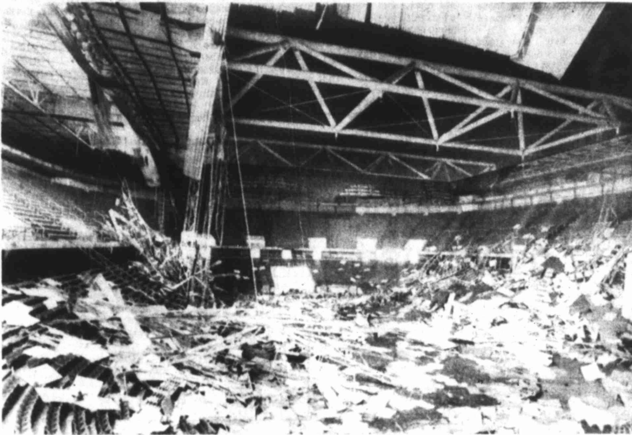
ROOF COLLAPSED — Nearly all of the roof of the 17,000-seat Kemper Arena in downtown Kansas City collapsed Monday night during a severe thunderstorm that dumped three inches of rain on the area in less than an hour and was accompanied by 70 mph winds. The arena, the site of the 1976 Republican National Convention, was not in use at the time of the collapse.
