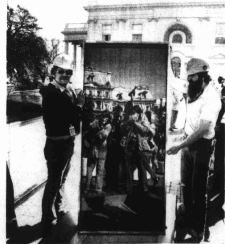
SOLAR COLLECTORS INSTALLED — Two workmen hold a solar panel on the roof of the White House Thursday during construction of a solar heating system to provide hot water for the Executive Mansion. Photographers and the Ole Executive Office Building are reflected in the bright surface of the panel.
