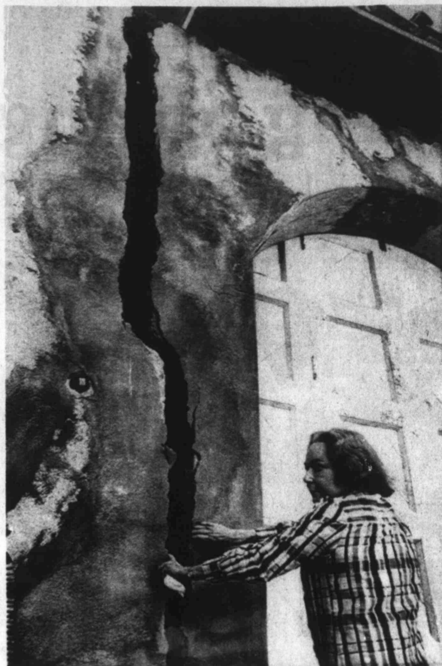
CRACKS ATTEST TO GROUND SLIPPAGE — Mrs. Betty Harden looks at the crack between her home and garage in the exclusive Portuguese Bend area where the slow slippage of the ground is damaging many homes in and around the neighborhood. The once, choice houses in the landslide area are now impossible to sell as banks will not make loans to prospective buyers. One owner says his $200,000 home is practically worthless.
