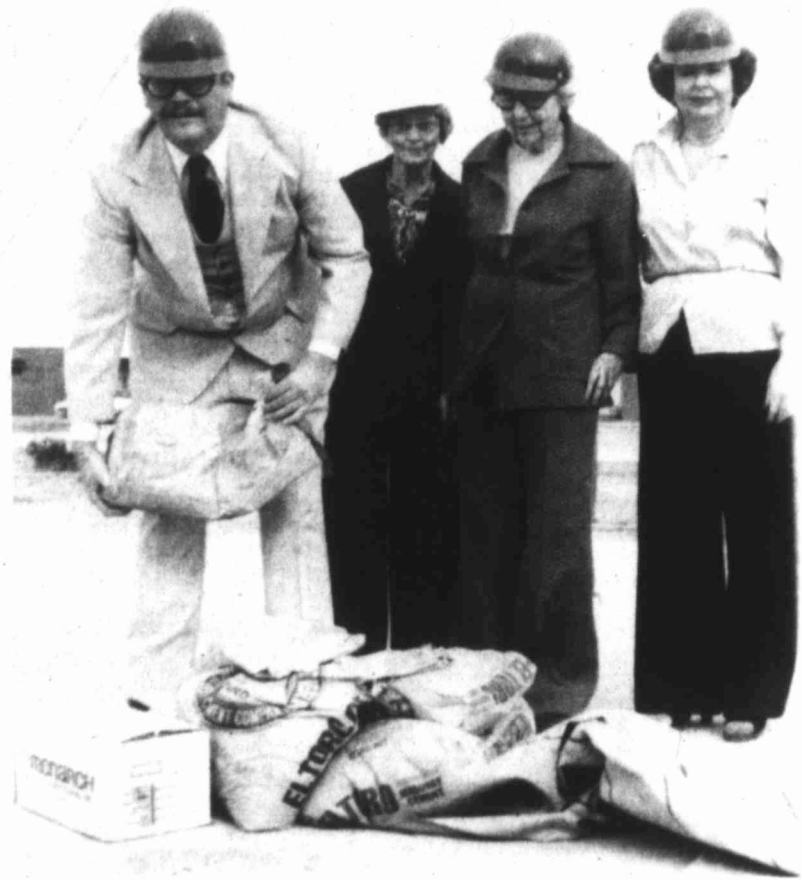
MIXING CEMENT — Before Chaparral Contractors could begin mixing the cement the new therapeutic swimming pool at BSSH funds had to be raised by members of the BSSH Volunteer Services Council. Pictured left to right are Lance Hays, Odessa; Mrs. Velma Bartlett, Lamesa; Mrs. R.M. Reed, Colorado City, Mitchell County Circuit Riders, clerk; and Mrs. John Caldwell, Midland.
