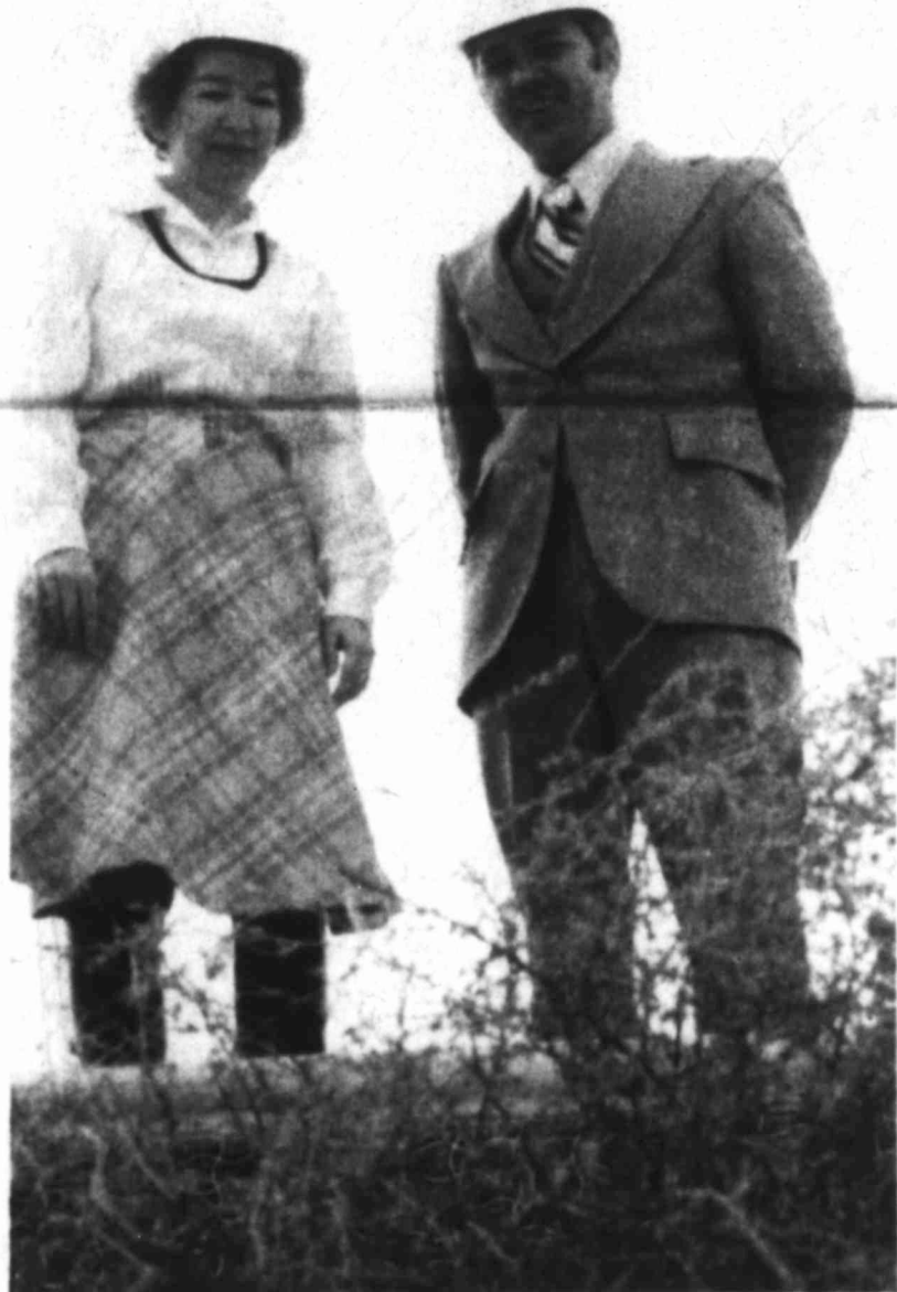
SOON WATER WILL REPLACE TUMBLEWEEDS — Here, Mrs. Shirley Shroyer, volunteer coordinator for BSSH, and Adolph Supak, assistant superintendent at BSSH, look into the partially completed therapeutic swimming pool. Both realize that by the middle of March, those tumbleweeds will be replaced with water, thanks to the tremendous effort put forth by the BSSH Volunteer Services Council to secure funds for construction.
