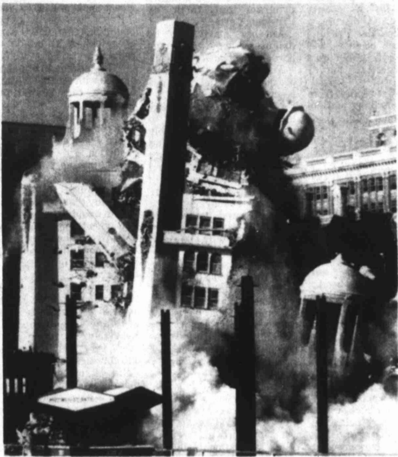
LANDMARK DEMOLISHED — The classic rotunda section of the Blenheim Hotel on the Boardwalk in Atlantic City, N.J. fell victim to this resort's casino era as it was demolished by dynamite blasts Thursday to make way for a $113 million dollar Casino hotel to be built by Bally Manufacturing, Inc. of Chicago.
