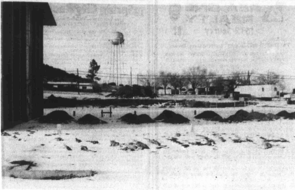
FOR THE NEXT DECADE — First Baptist Church has set the first part of 1980 as the goal for completion of a million dollar building on which construction has begun at 705 W. Marcy. The building is being constructed in order to provide additional activities for youth and children, according to Ron Killough, Minister of Education at the church. It will include a chapel with a
