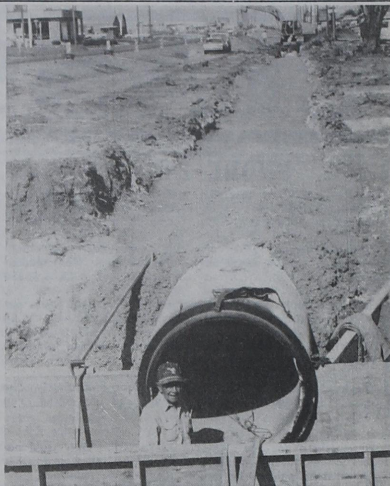
NEW DRAIN PIPE.... A new storm drain is being installed for the Highway 60 widening project through Friona. A workman is shown on West Highway 60. (Photo by Lisa McLellan)
