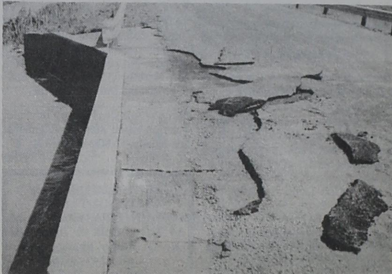
APPARENT DAMAGE....Water apparently overflowed this culvert causing part of the asphalt to wash out as Frio Draw raged for the first time in several years.
