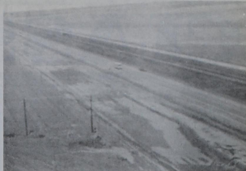
ROAD DAMAGE....Approximately two miles of caliche was washed away on the new stretch of Highway 60 east of Bovina.
