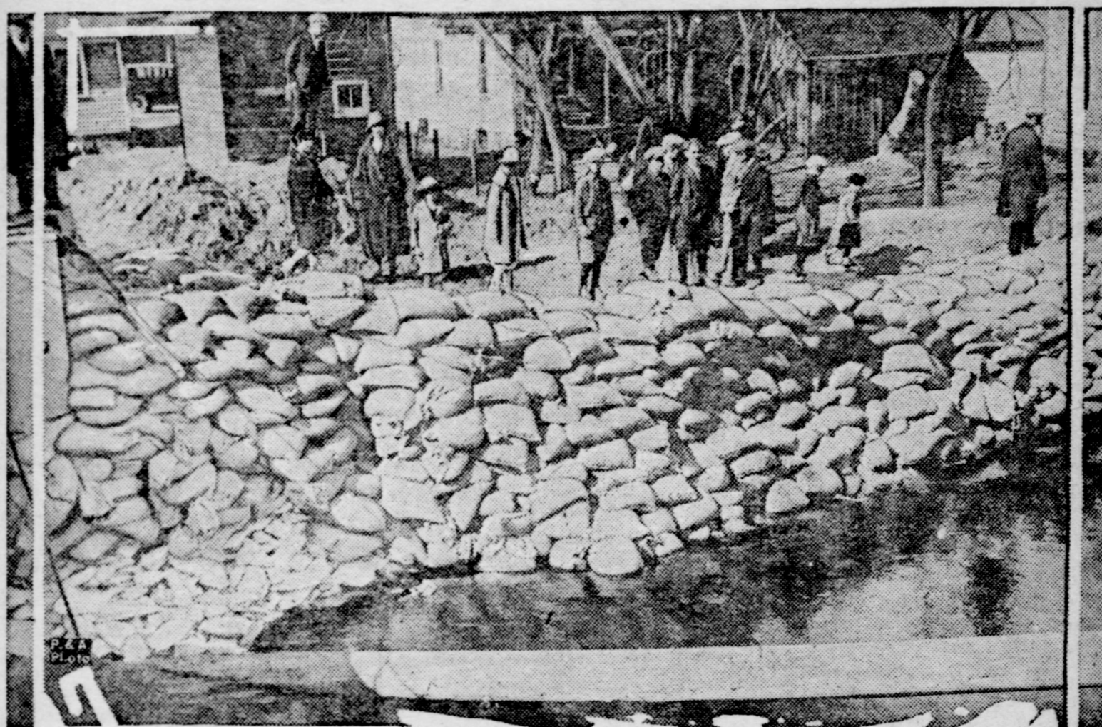
After an all-night fight, residents of Portage, Wis., succeeded in blocking a break in the wall of a canal between the Fox and Wisconsin rivers, and saved the town from an imminent flood. The high waters forced down seventy-five feet of the wall, and weakened the gates at the Wisconsin river end of the canal. Citizens filled the gap with granite and sandbags.
