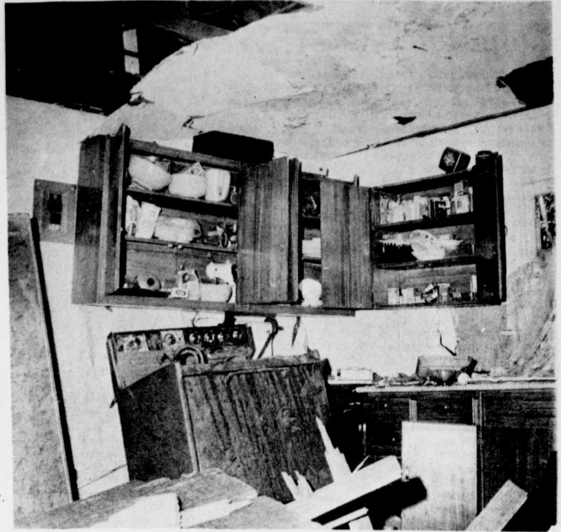
TILTED STOVE AND DEBRIS--This is a graphic illustration of the damage sustained at the M. W. Vise home near Clay's Corner Friday morning. The tilted stove was flung away from the wall as the floor exploded upward. Irvin St. Clair, who owned the farm home, said he considered the home a total loss in the mid-morning explosion.
