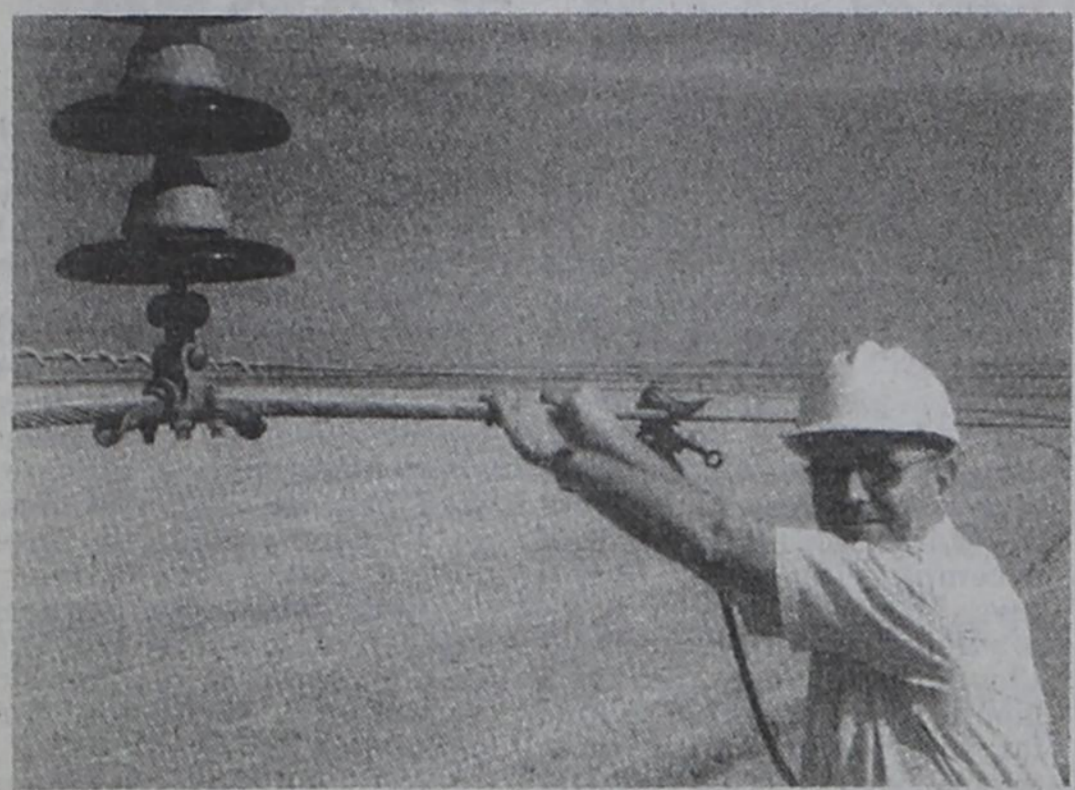
TOMMIE WEEMES , DSEC's member services manager, grips the energized 69,000-volt transmission line. Although this is not exactly in his job description, he did it to research the article and to experience some of the techniques of bare-handing high-voltage lines.
