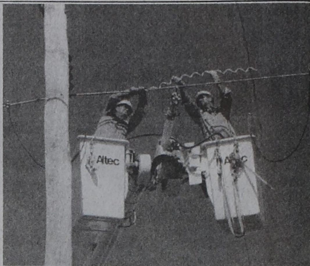
HIGH VOLTAGE CREW... DSEC's high-voltage crew, Harold Finch (left) and Bruce Johnson, install vibration dampers on an energized 69,000-volt transmission line. The dampers are installed to prevent wire damage from wind vibration. The wire on this line was damaged and required splicing in several places. The new bucket truck was designed to allow the crew to work using bare-hand techniques on the energized high-voltage transmission line.
