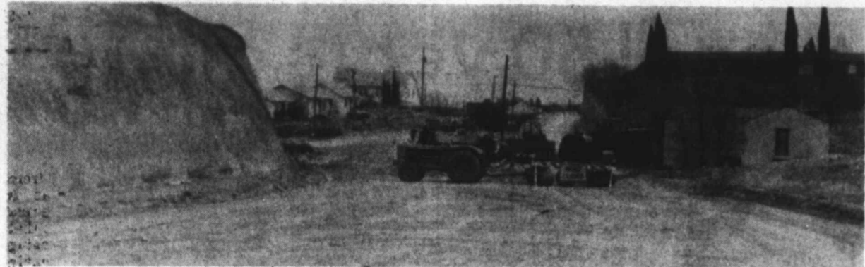
CONSTRUCTION UNDER WAY — The 11th Place Extension from in front of the Malone-Hogan Hospital to Gregg street is now underway. The street will come out at 10th Street at Gregg. This will connect FM 700 and Gregg Street and relieve traffic on both arteries. Funding was through the state highway department.
