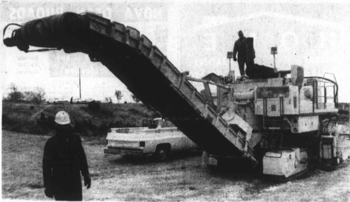
OFF THE TOP — The State Department of Highways contracted to bring in this Rotar Mill from C.M.I. in Oklahoma City to both roughen up and smooth up some of the local highways. It was used on FM 700 and other locations to take the top off of knots in the pavement
