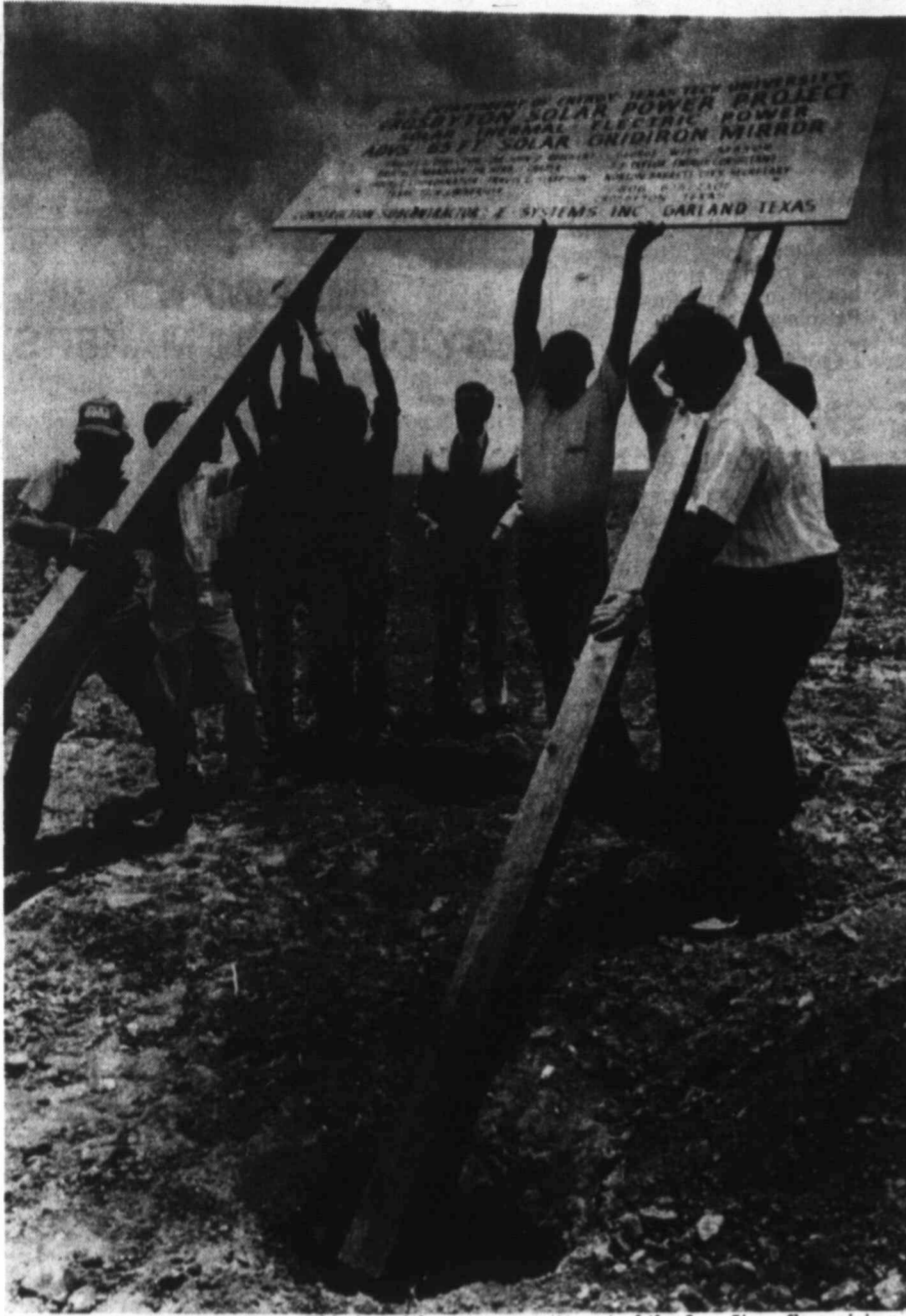
SIGN OF THE TIMES — This is neither a re-enactment of the two Jima flagraising nor training for destruction of football goalposts. But there is just as much excitement as Crosbyton, officials and employees erect a sign designating a 10-acre test site for the 65-foot diameter, spherical shaped solar energy collector to be built in the West Texas farm community.
