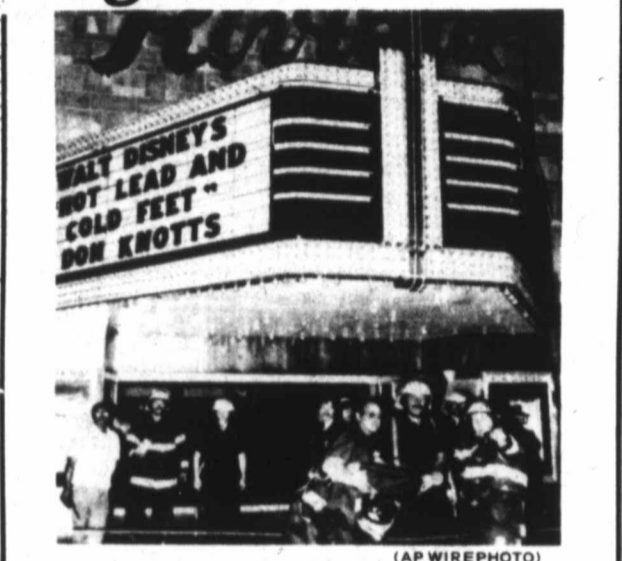
THREE INJURED — Anderson, Indiana, firemen stand outside the Riviera movie theater that had its roof collapse injuring three persons due to heavy rains Sunday night. Between 100 and 150 people were inside when the water poured in.
