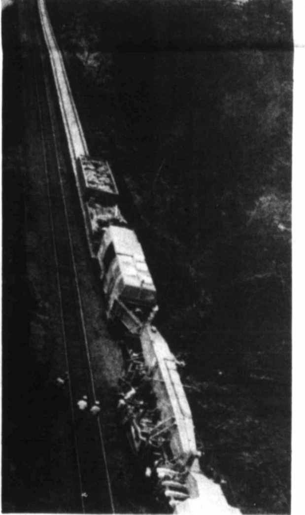
NEW RAILROAD — With a path of new white concrete ties leaving a clear path behind the 95-ton track laying machine moves slowly forward as it replaces old wooden ties and rails at a mile-a-day pace. The machine and support cars stretch along the track for a quarter of a mile and employ a crew of 160 persons.
