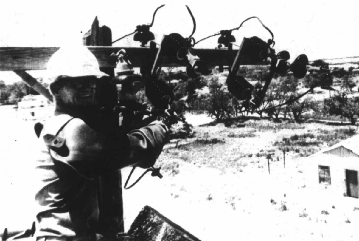
THE WEST TEXAS LINEMAN — A.W. Henry, with 24 years experience, is still on the line for Texas Electric. Henry is working on a West 3rd St. project, replacing poles and conductors from Alfred St. to Jones St. The old copper wiring is being replaced with aluminum conductor steel-reinforced (ACSR). The copper had been in service since the 30s, but in three weeks the project will replace most of it.
