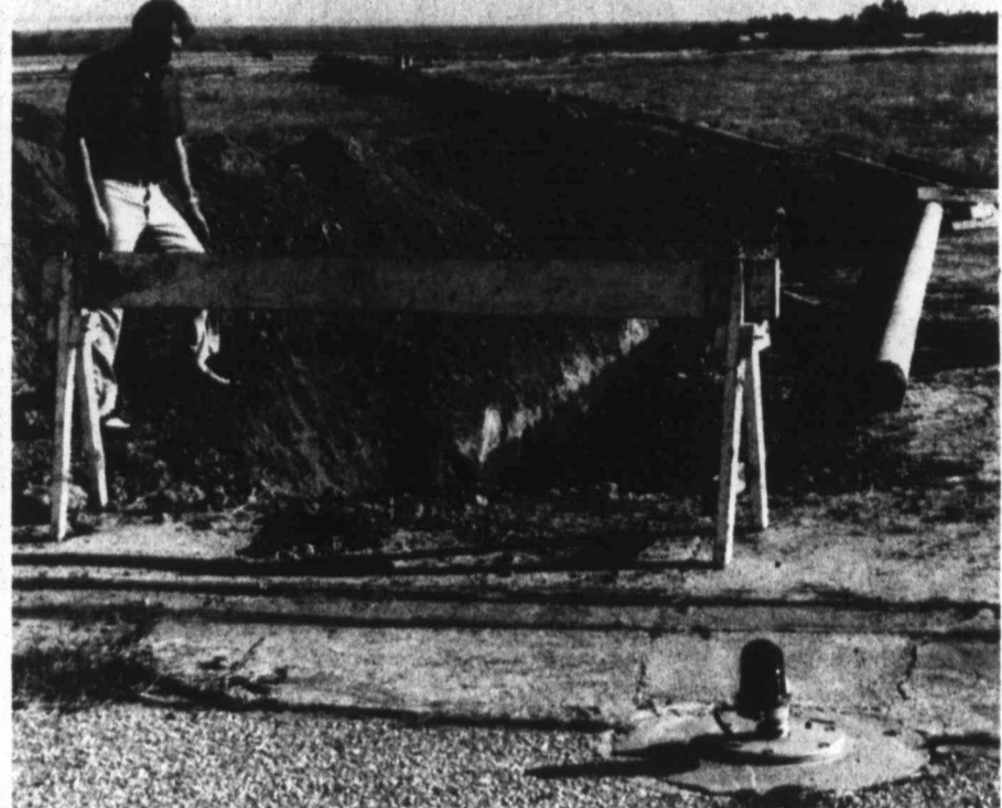
NEW WATER LINE — Harry Spannaus, industrial park manager, is shown checking out the new pipeline being built by Cosden to connect water wells at Webb golf course to the fuel line into Cosden so that water may be sold to the Cosden Asphalt plant. Revenue from the water sale will go to the city.
