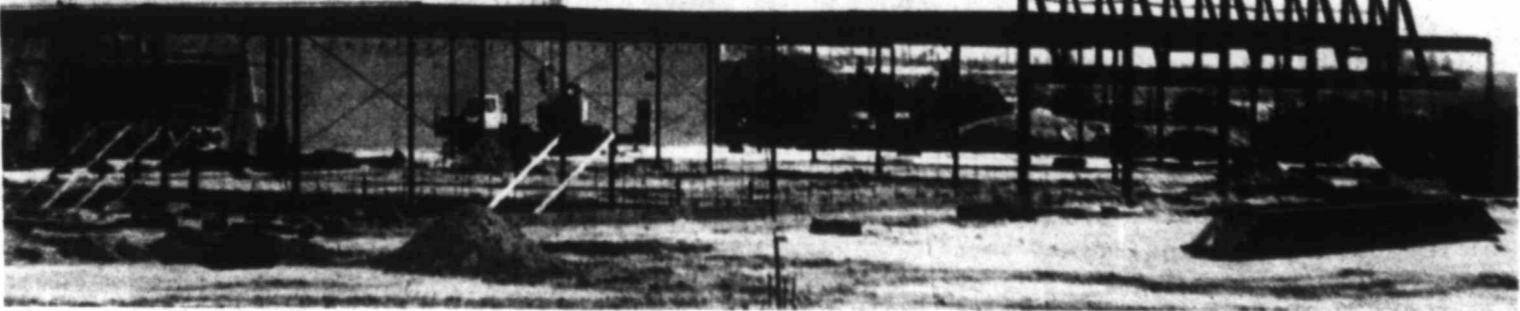
GOING UP — K-Mart is going up at its location east of Birdwell near FM 700. The new business is expected to be complete sometime in the fall and add to the fast growing business area near or on FM 700 from Gollad east. (PHOTO BY DANNY VALDES)
