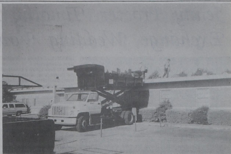
HOT WORK.....Parmer County Community Hospital will soon have work completed on a new roof. Fortunately for the workers, in case of heat problems, help is just below.
