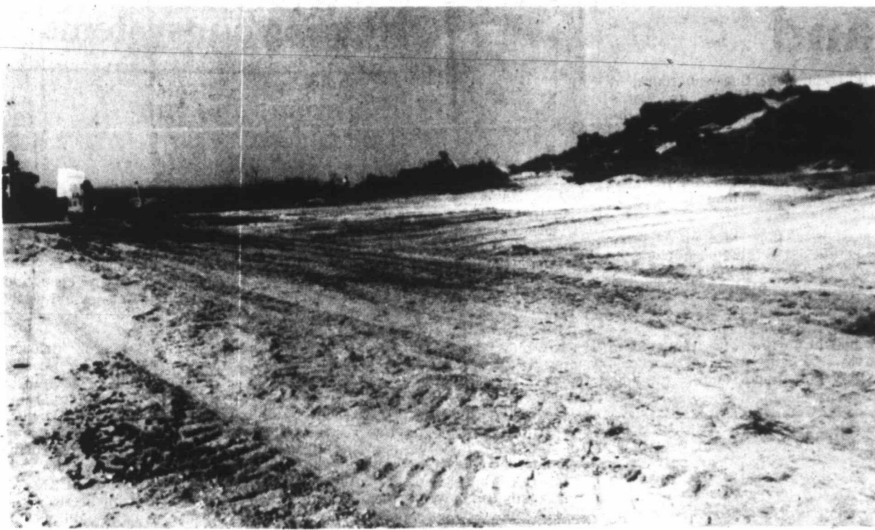
CLEARING FOR SKATE BOARDS — The skate board park will soon become a reality on FM 700 with clearing of the land and a layout with lines for the project under way here Tuesday. The proposed park caused a zoning disagreement earlier in the year, but has been anxiously awaited by local skate board enthusiasts.
