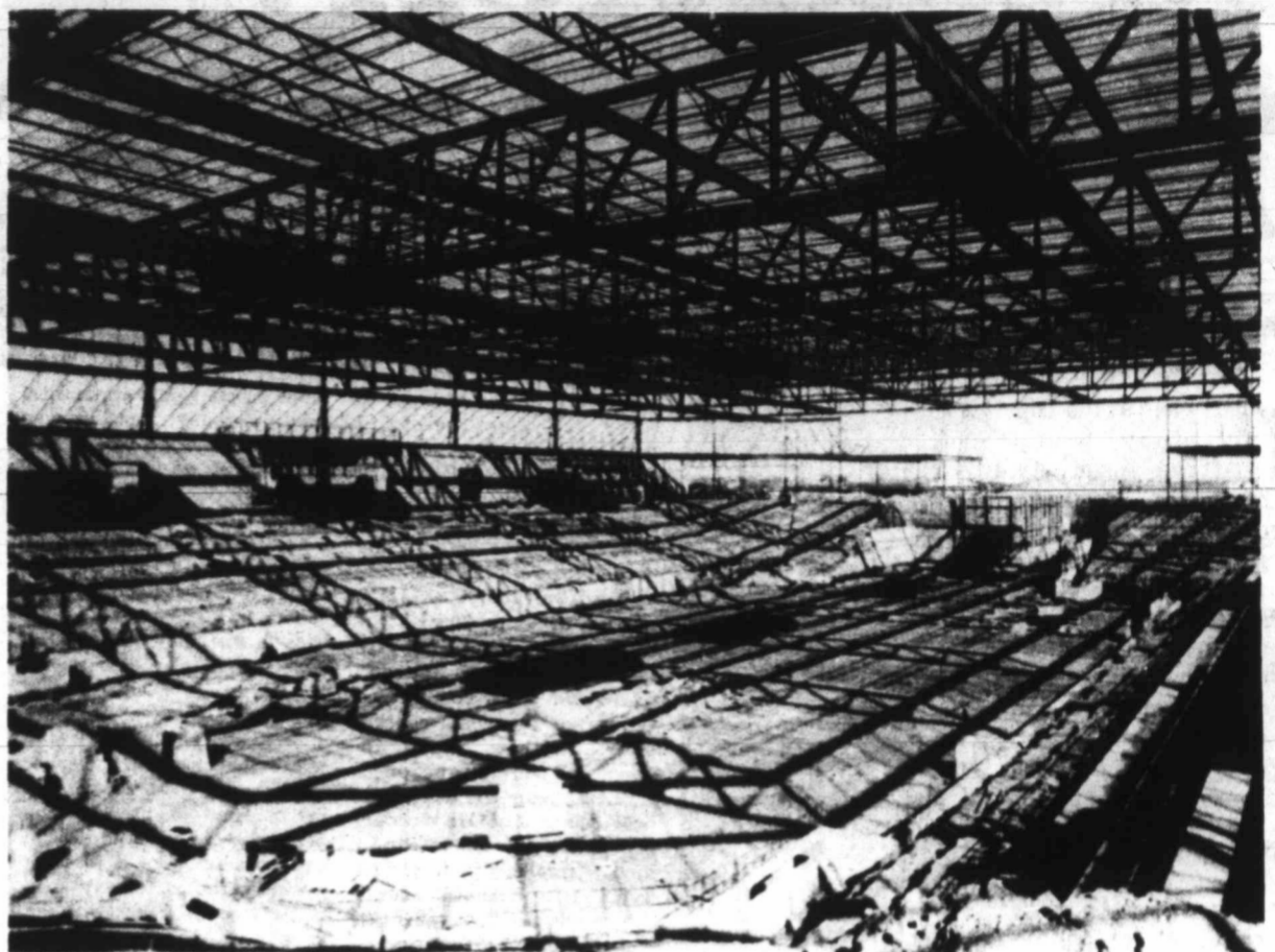
GOING, GOING, GOING — The coliseum has been going up for many months since ground was broken in March 1976 and it looks as though
