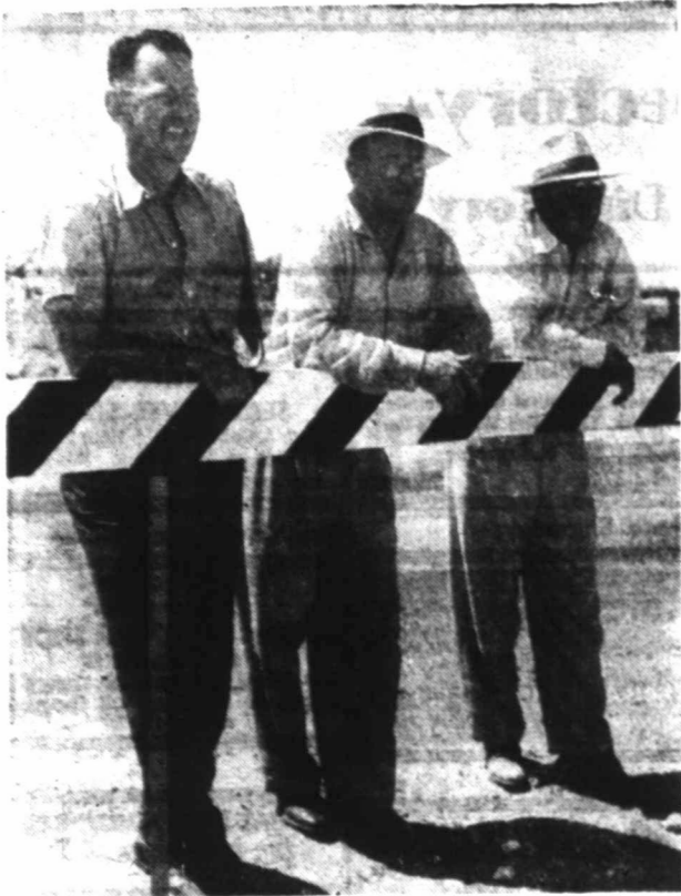
NOT JUST SPECTATORS —These men shown watching pipe line construction are far from just mildly interested spectators. All three have a hand in the million-dollar operation. Left to right are H. K. Miller, general inspector, and R. D. Schollenbarger, chief inspector, for Permian Basin Pipeline Company, and M. L. Boyd, Fulton Company superintendent.
