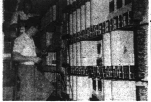
CONNECTIONS SOLDERED —Western Electric workers solder connections in Stanton's new dial telephone building.
