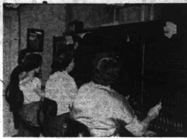
OLD SWITCHBOARD —Stanton operators are shown at the manual switchboard which soon will pass out of the picture. The operators are Mamie McDurmon, chief; Sybil Bickley, Dorothy Cline and Cecil White.
