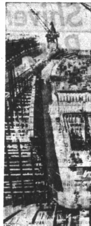
GROWTH OF A SUPERCARRIER—Covered by a framework of steel girders and hovering derricks, the keel of the controversial U.S.S. Forrestal, started on July 14, is making rapid progress.
