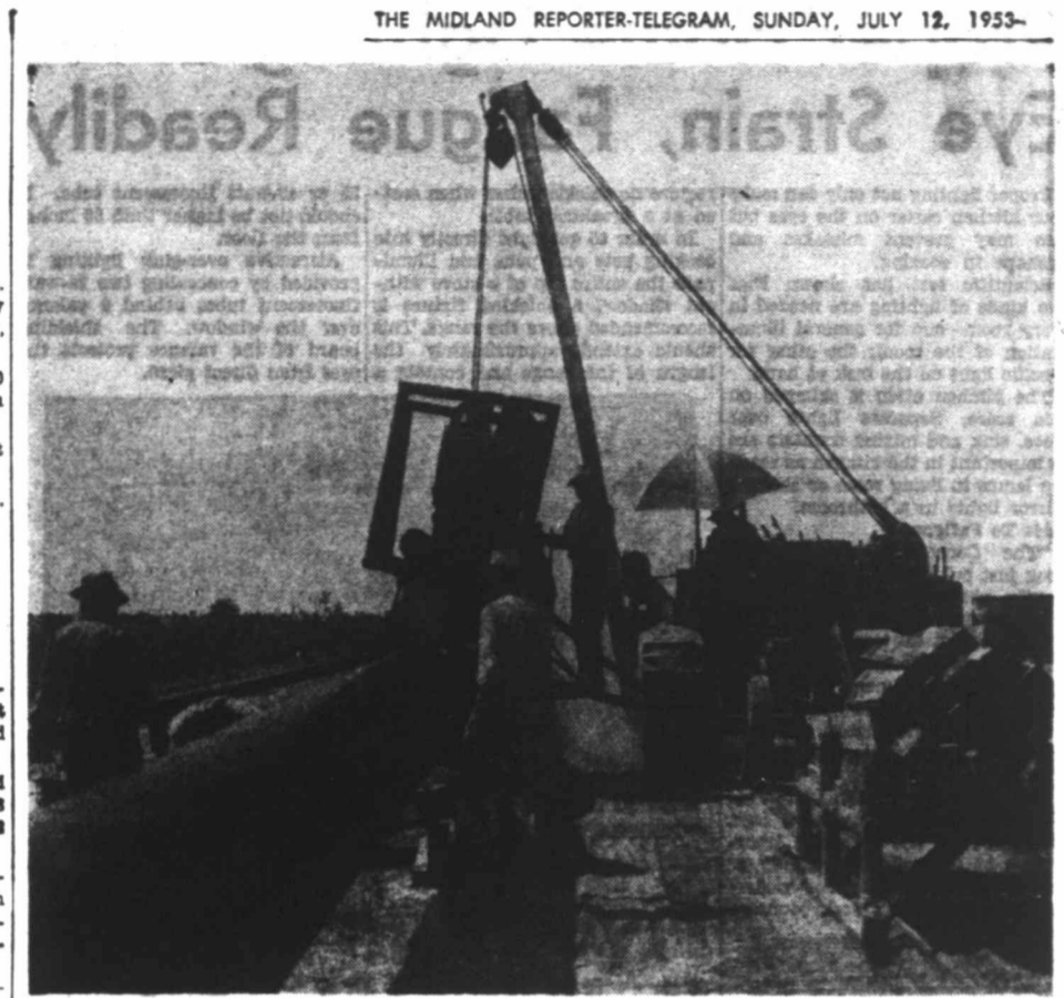
PIPE GETS ITS WRAPPING — Part of the Permian Basin Pipeline Company's pipe line through the Spraberry Trend Area gets "gift wrapped" by workers and machines of the R. H. Fulton Company. It's "gift wrapping" because the pipe will soon be taking residue gas from the Spraberry Area thus netting neat profits for all concerned and dulling the danger of shutoff actions.
