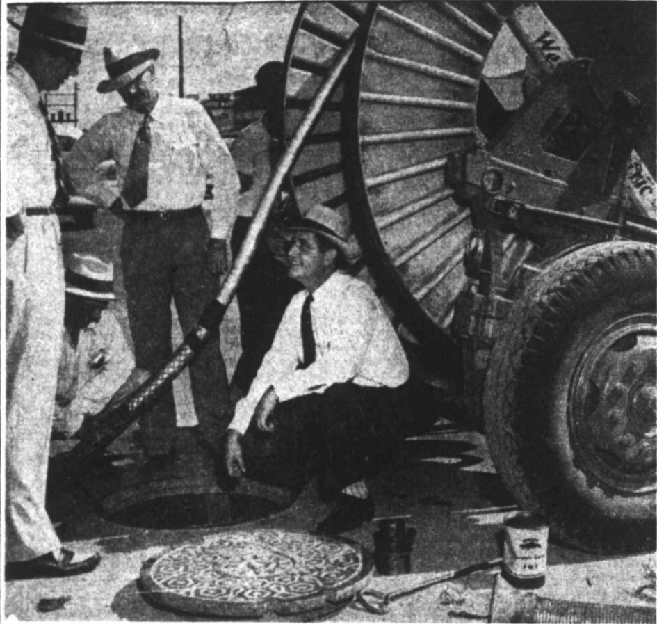
EXPANSION PROGRAM —Work is underway in the expansion program of the Southwestern Bell Telephone Company, which will result in telephone service for the Permian Estates area in West Midland. Here a group of telephone company employes watch new cable go into a manhole on West Wall Street. Left to right: Bill Yeatts, district manager; Wade Atteaway, foreman; H. H. Nicholson, supervisor, and Dave Dillard, Midland manager. The employe standing behind the reel was not identified. (See story Page 16.)
