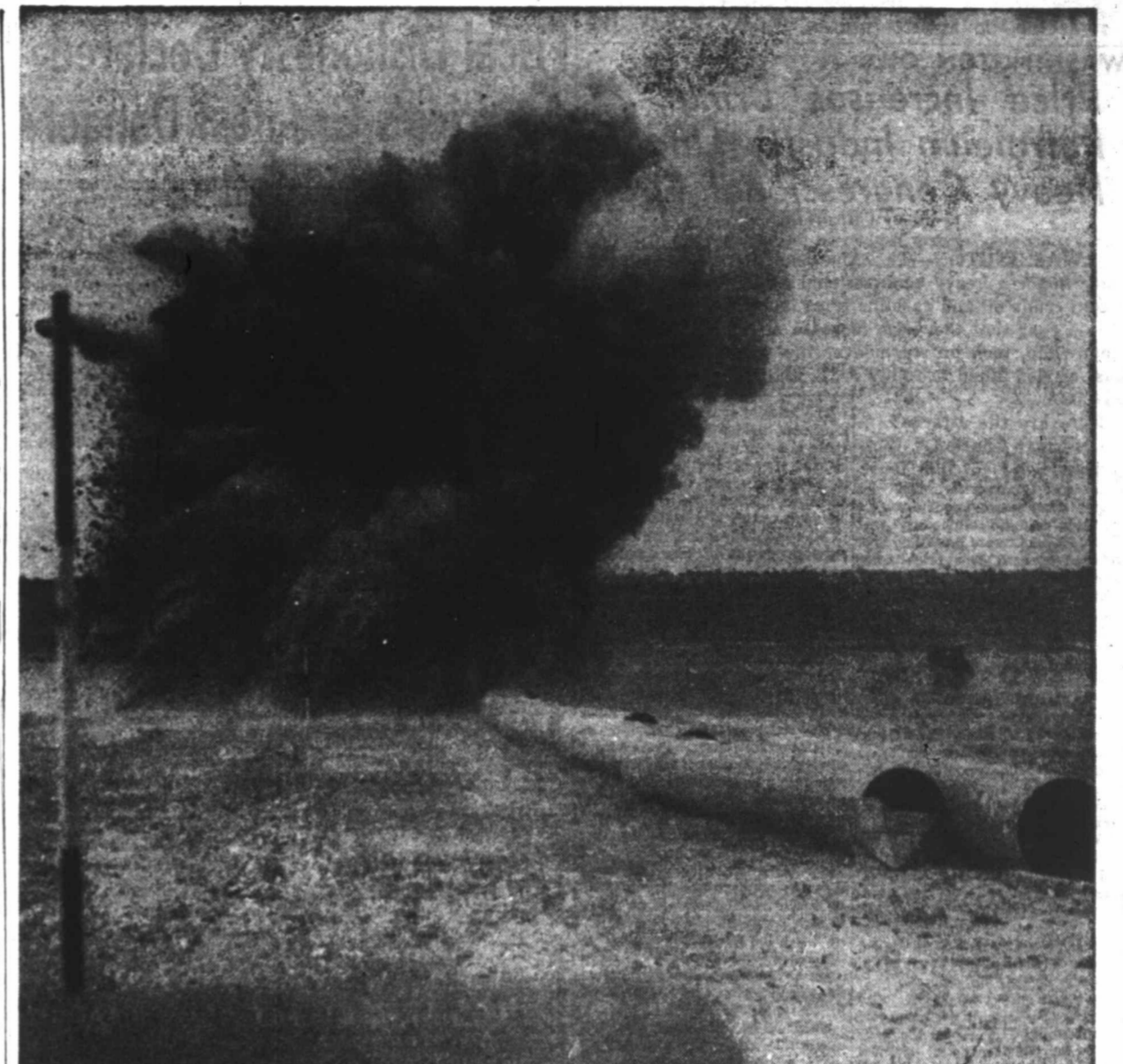
THE BOOM'S CLOSER TO MIDLAND—The boom and crash of before-digger blasts moved closer to Midland last week as work continued as a fast clip on the 285-mile Permian Basin Pipeline Company's line destined to remove much of the residue gas from
