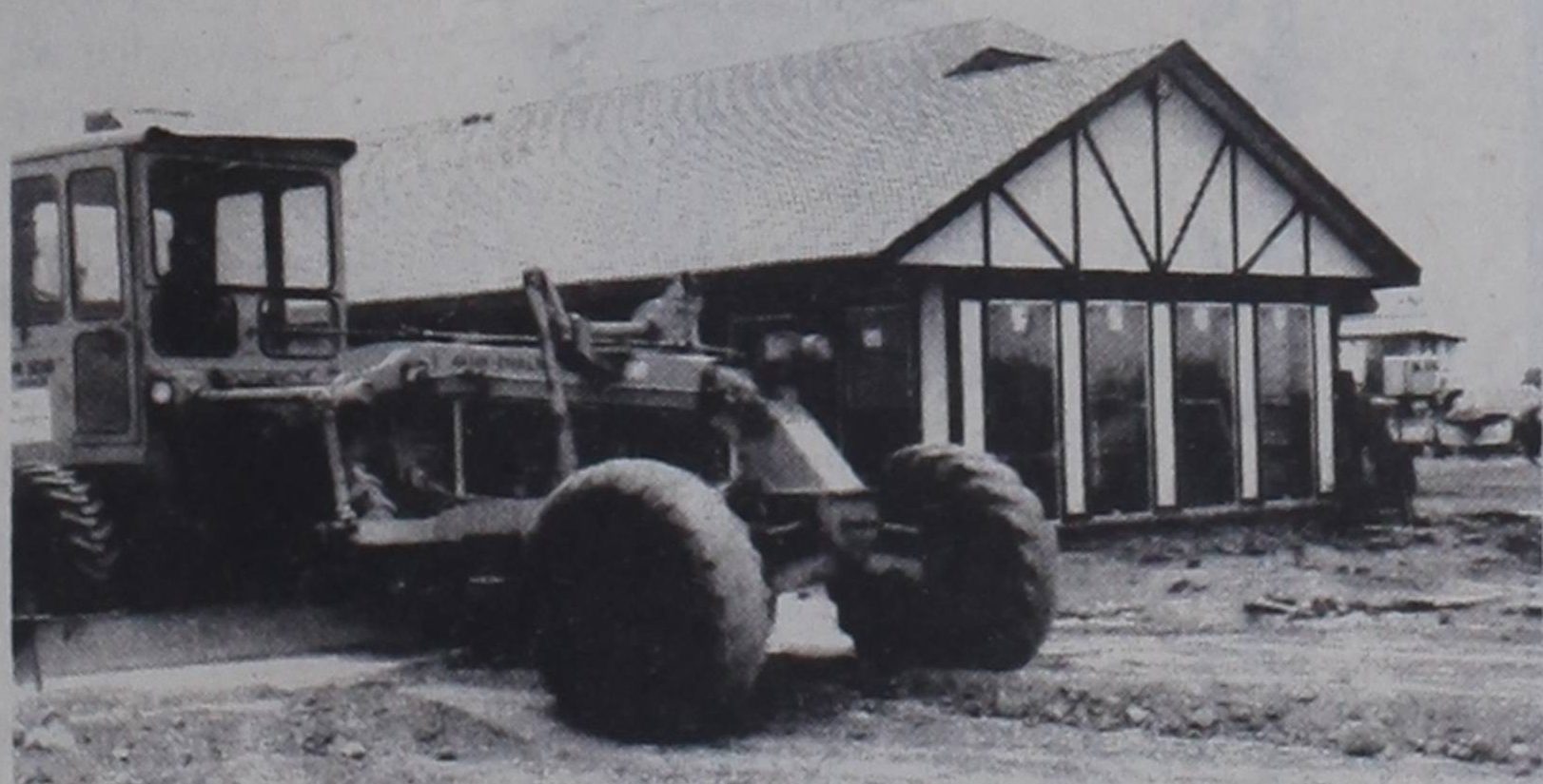
WORK CONTINUES... The new motel on West Highway 60 has taken shape fairly rapidly, and according to the Chamber of Commerce, will be open for pheasant season's opening weekend.
