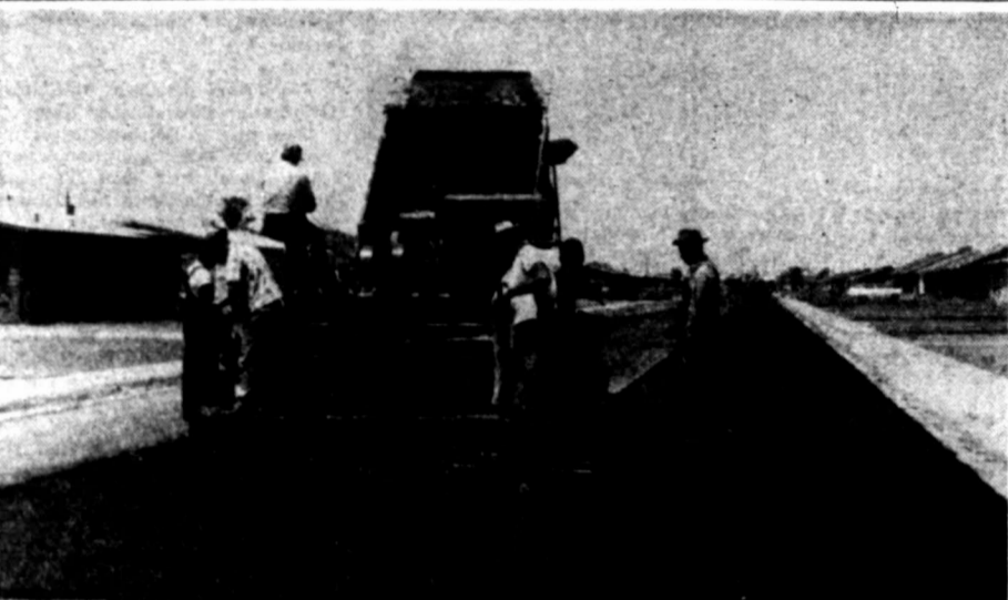
FINAL PAVING ON 200-BLOCK PROJECT STARTED—A huge asphalt spreader begins the job of laying a finished surface for the current 200-block paving project.
