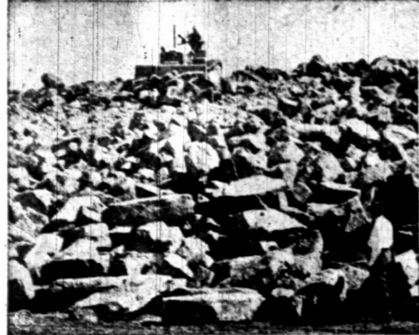
Meanwhile work continues at Tuttle Creek, where 850,000 cubic yards of rock fill have been placed. National administration's...
