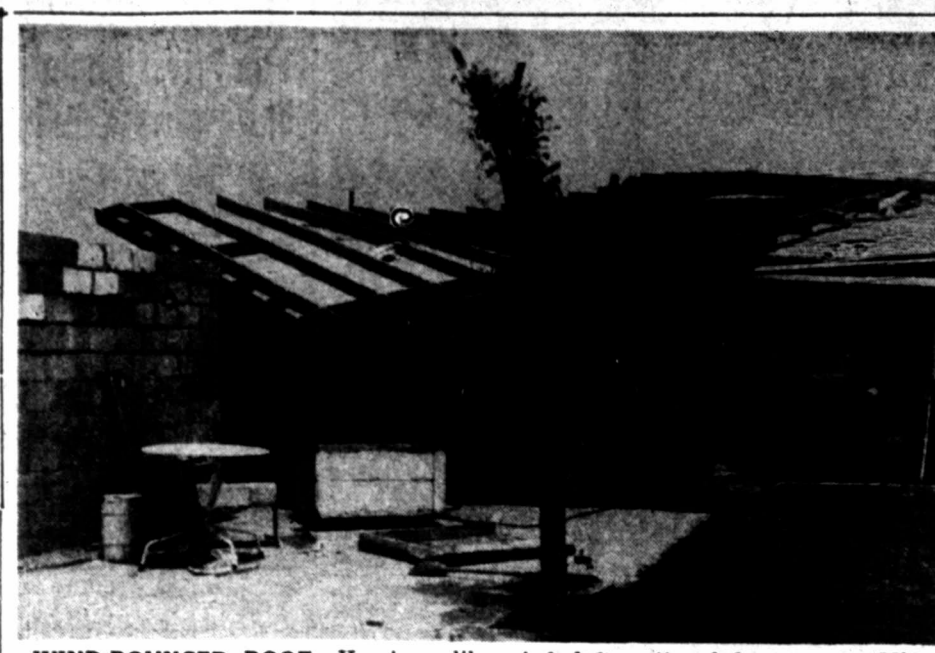
WIND-BOUNCED ROOF —Hurricane-like winds left scattered damage over Midland and the Permian Basin this week. Major loss occurred at this residence on North Big Spring Street. The roof of the adjoining garage was ripped off and flipped onto the top of the house. It tore a large hole in the roof of the residence. Other damage to roofs, carts, television towers, fences, trees and shrubbery was reported over the city Thursday after the two-day gales subsided.
